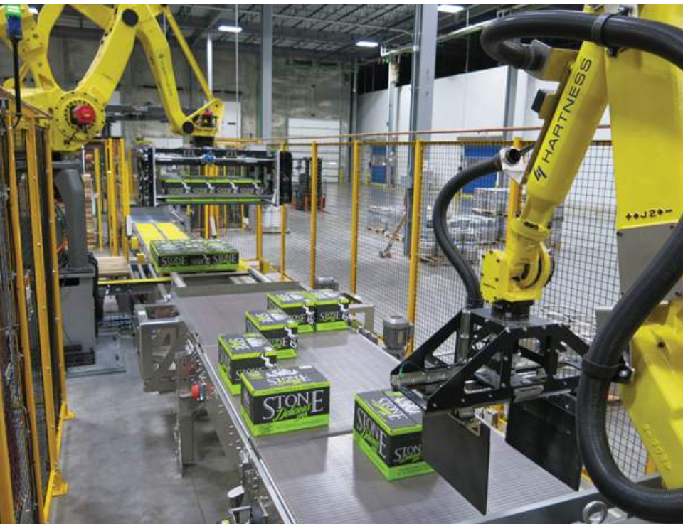
A robotic palletizer and stretch wrapper reside at the end of the line.
