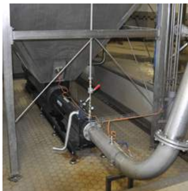
A progressing cavity pump is used at Victory Brewing to pump spent grain to outdoor silos.
